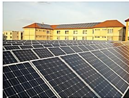
RES installation on several municipal buildings in Alba Iulia (PV solar) - Copyright: ALEA
